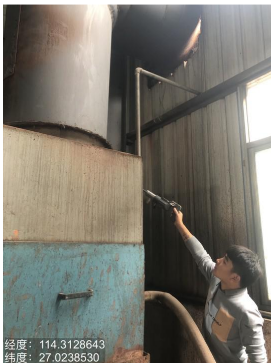
喷涂废气进口1#
